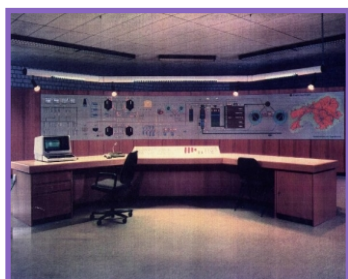
Main Control Room
